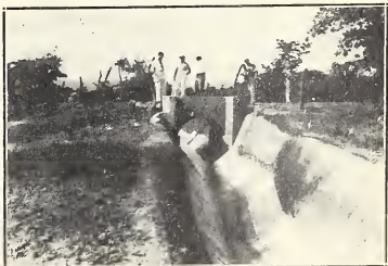
Fig. 5. This ditch at Santiago, in the Republic of Cuba, is lined with thirds of concrete pipe 36 inches in diameter instead of inverts.
